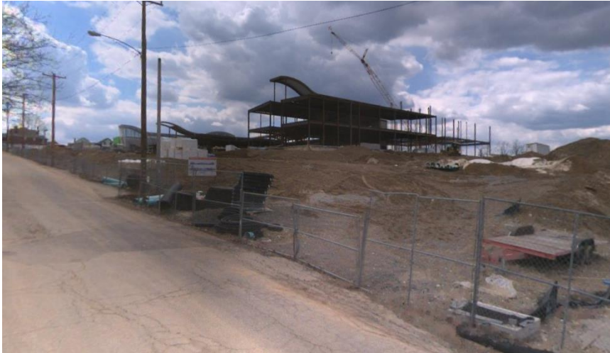
Figure 21 Neighboring Street with Soil Washoff
